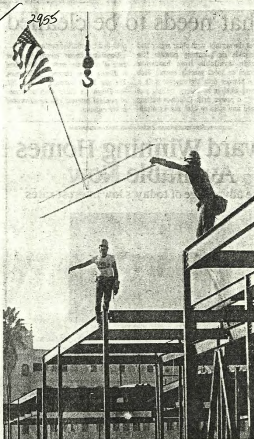
Old Glory: A flag flies from the last of 3,972 steel beams installed recently at University Center on the University of San Diego campus. The $9 million so-called campus "living room" contains nearly 500 tons of steel beams, said Paul Muzzy, marketing director for Trepte Construction Co. USD president Author E. Hughes and others added their signatures to the beam before it was placed in the 74,500-square-foot, two-level structure which features a student dining hall, faculty dining room, student government offices, deli and sundries store. It is the fourth multi-million dollar building to rise on the campus since 1983.
