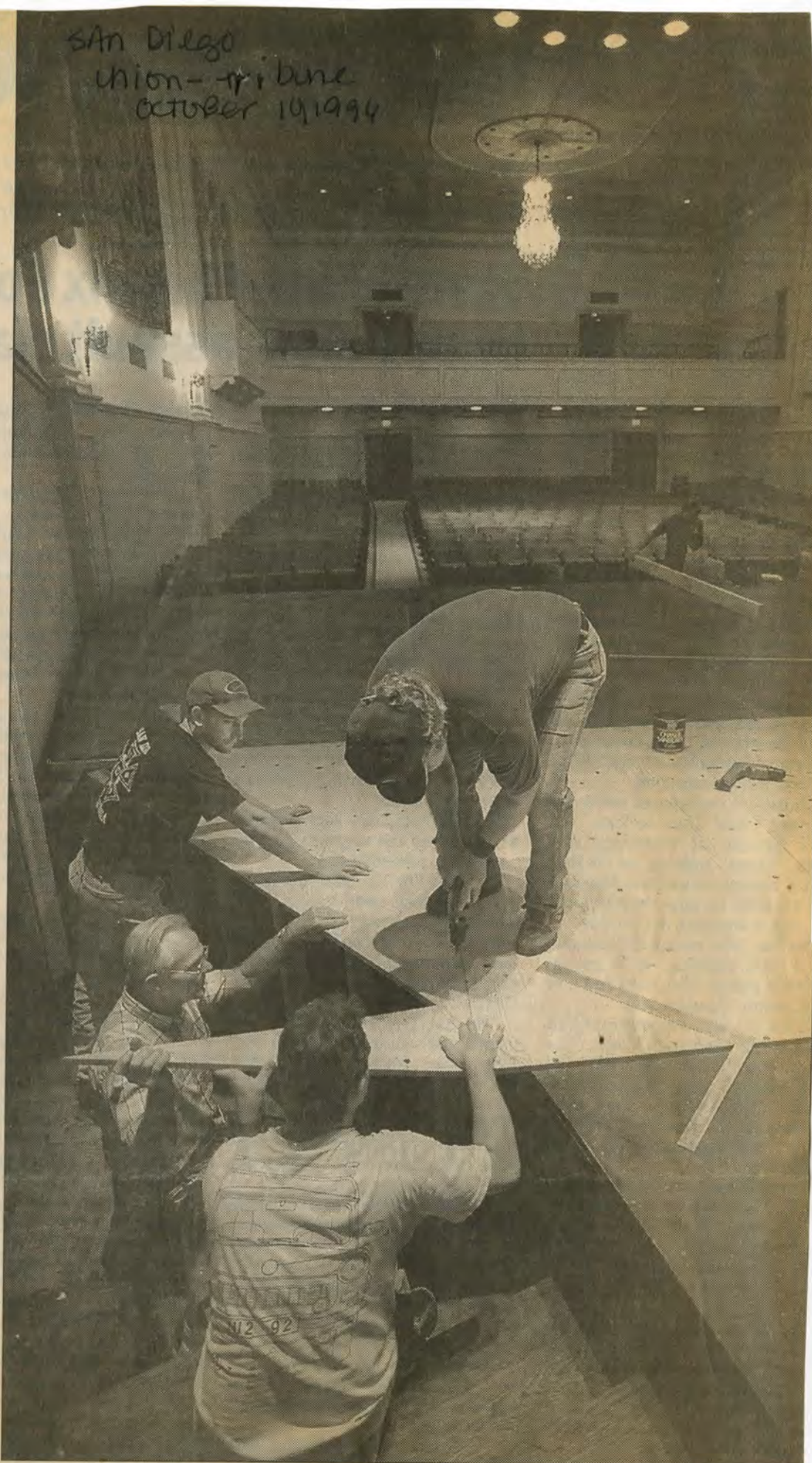
Hard at work: A crew builds the platform for Wednesday's debate. Counterclockwise are Fred Nace (with drill), Trevor Hay, Gene Reilly and John Kenniston. 54
