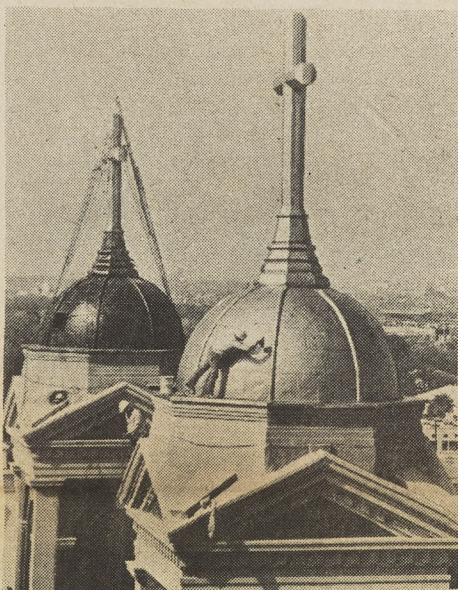
Passersby are encouraged to wear dark glasses as they glance up 150 feet at the twin domes of Immaculate Conception Cathedral in Mobile, Ala. A gold epoxy is being painted on which should retain its brightness for at least 20 years.
