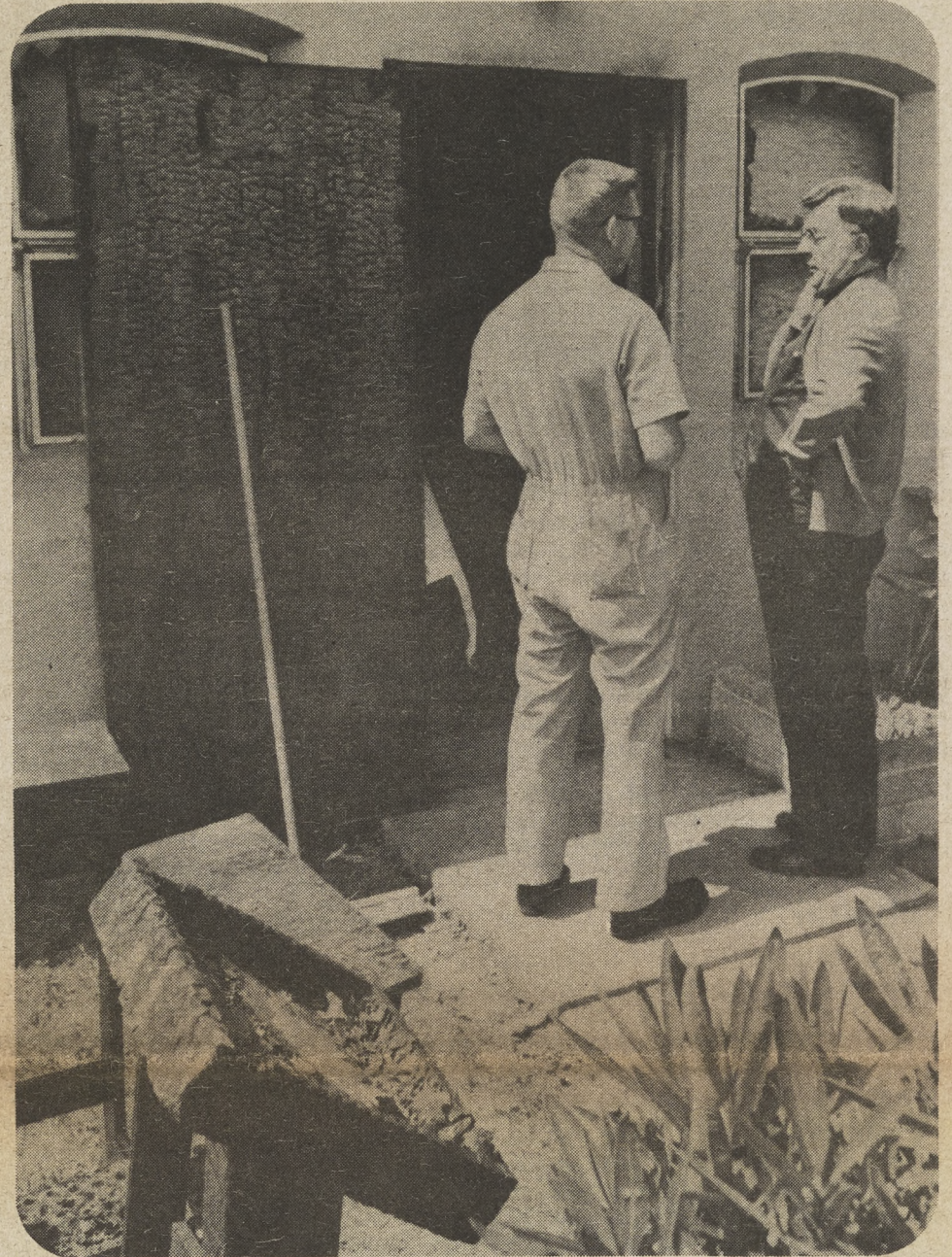
FIRE DAMAGE —Msgr. Sean Murray, right, pastor of St. Therese, San Diego, talks to parish custodian Andy Fekete in front of the charred door and broken windows of the altar boys' sacristy of the church. On April 25, an arsonist
