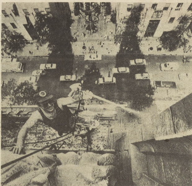
CENTURY OF DIRT —Odilon Cerat of Tuper Lake, N.Y., sprays high pressure water on the front of St. Patrick Cathedral in New York City. Far below him is Fifth Avenue and Rockefeller Center. The cathedral, which is 100 years old this year, has been undergoing a major exterior cleaning. (NC photo)
